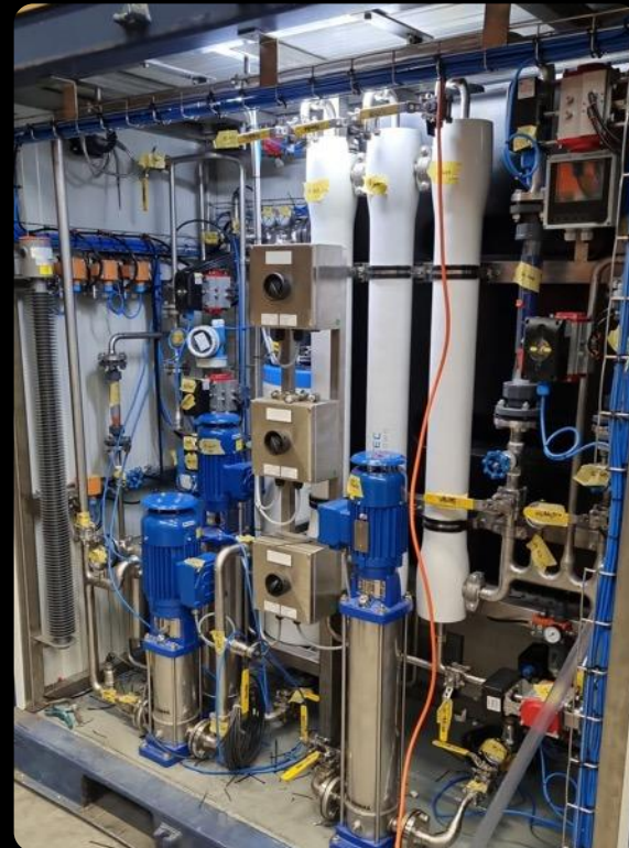
Containerized RO system for Demin water system for LNG plant
