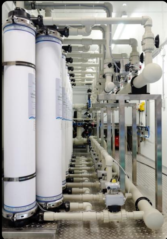
Containerized ultrafiltration unit Naval application
