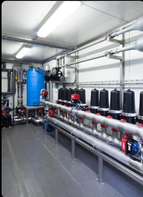
Side filtration with vortex cavitation system to eliminate calcium in cooling water applications
